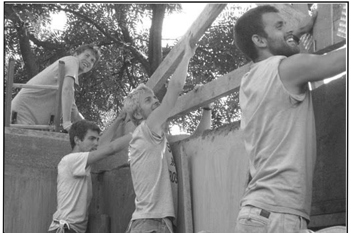
ISLA construction team members more than held their own, completing two school roofs during the January trip. Photo by Nancy Carlson
