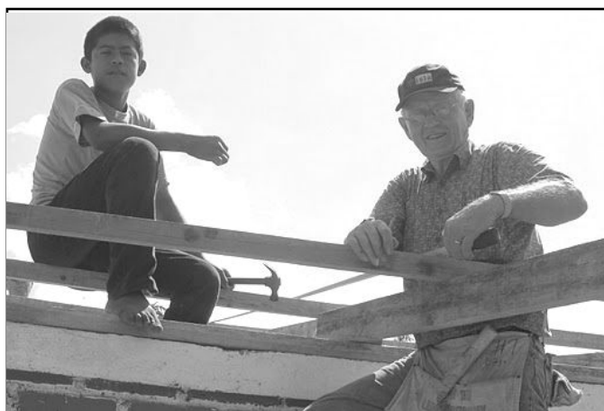
Bill Lindstrom (right) and other ISLA volunteers had plenty of help from locals in rebuilding roof projects. Photo by Nancy Carlson
